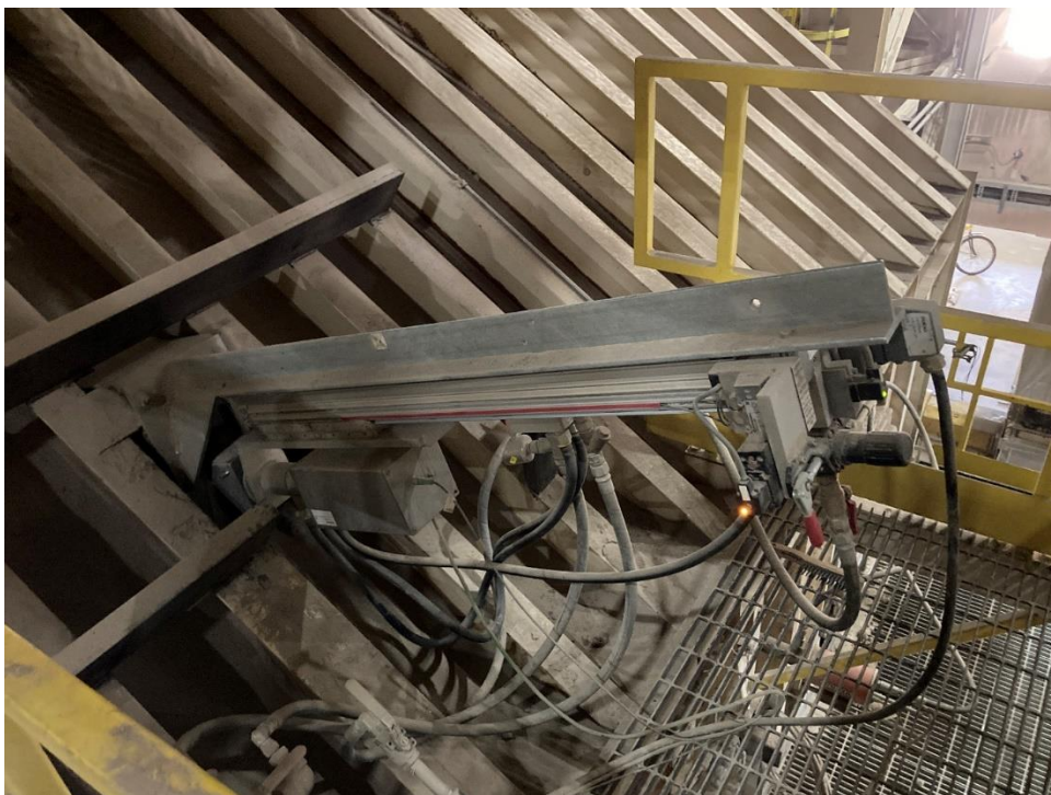
Figure 4 Installation in Grande Prairie, Alberta Canada
